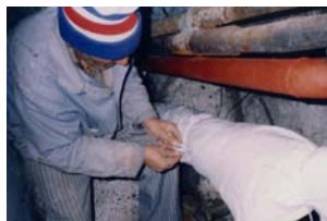
Insulation of drinking water pipes
