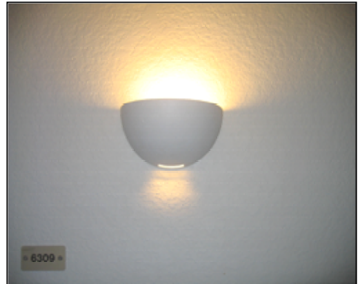
Wall mounted sconce to be removed.
